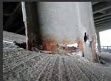
H-piling with major loss of web section due to corrosion
