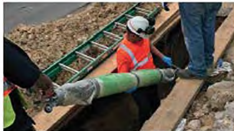
...before the repaired pipe was capped and tested under internal fluid pressure
