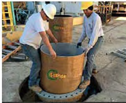
Insertion of StifPipe® into a Pressure Pipe Manhole at a Puerto Rico Power Plant
